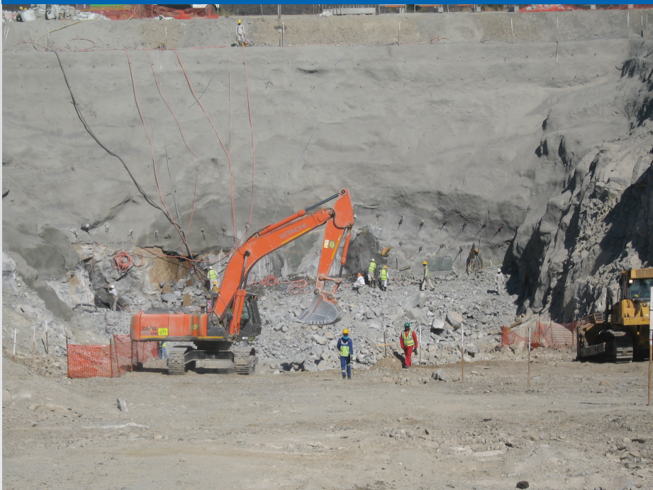
Photo, above: WBJV Project 1 Central Decline Box Cut, ready for start of Underground Development.
